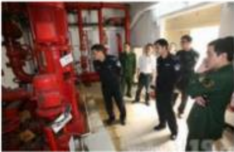
Firefighting facility issues
