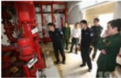
Firefighting facility issues
